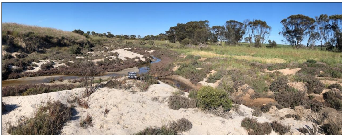
Figure 9: Warperup Creek floodway showing extensive sand plumes, eroded banks, fragmented tree and shrub cover with grasses and Samphire dominating.
